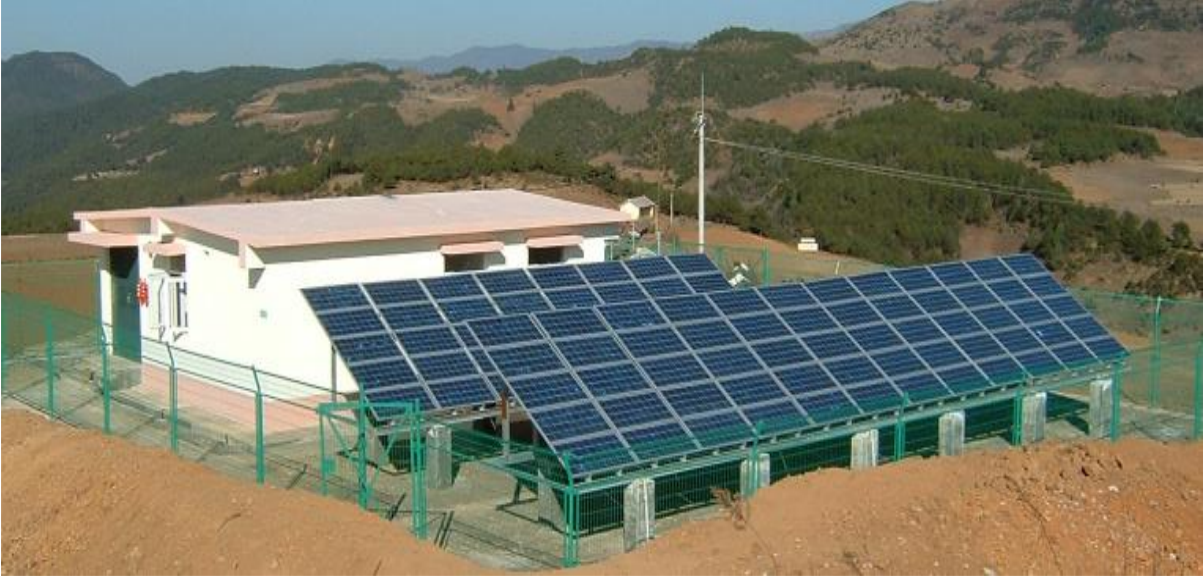
Figure 2 Solar PV Array and Battery/Genset Building
