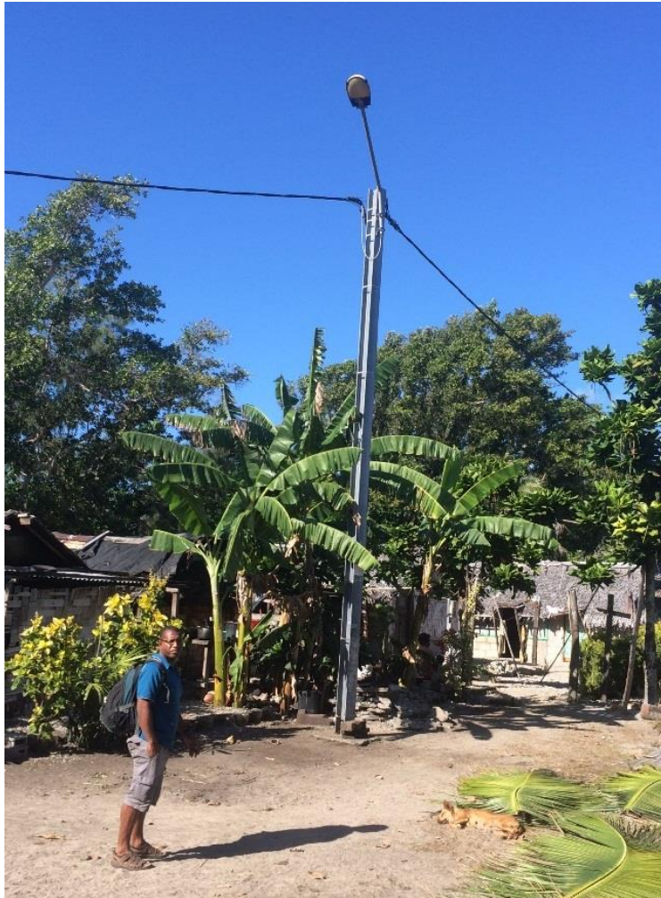
Figure 3 Power Pole and Distribution Lines
